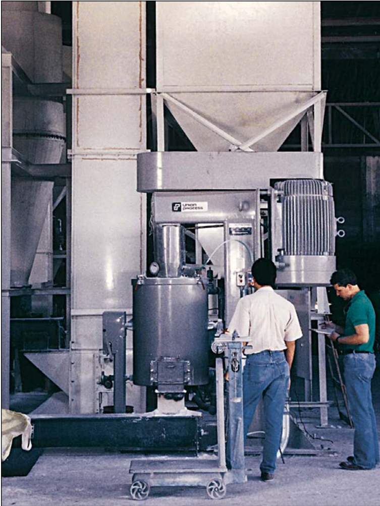
Installation of an HSA-100 for continuous fine dry grinding of calcium carbonate and barites.
